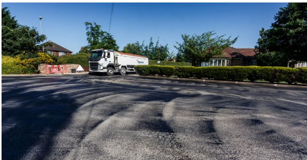
138 tonnes of asphalt supplied and laid free of charge for Wakefield hospice
