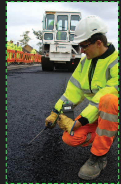
Hanson was the first company in the UK to produce and lay ERA (Energy Reducing Asphalt).
